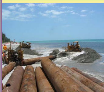
Sand being pumped onto the beach and spread by bulldozers at the last Captiva nourishment in 2005-06.
